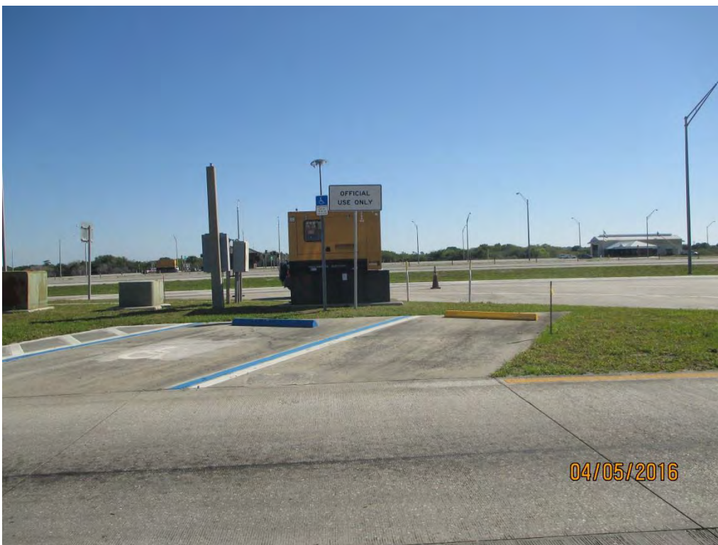
View to the east of emergency generator located adjacent to SB-WIM
